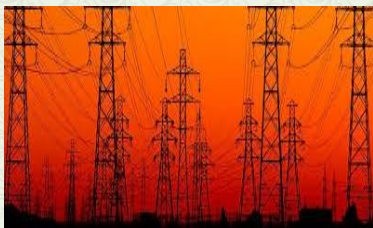
Power Generation, Transmission and Distribution
